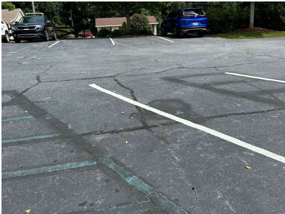
2. View of linear cracks at clubhouse parking lot.
