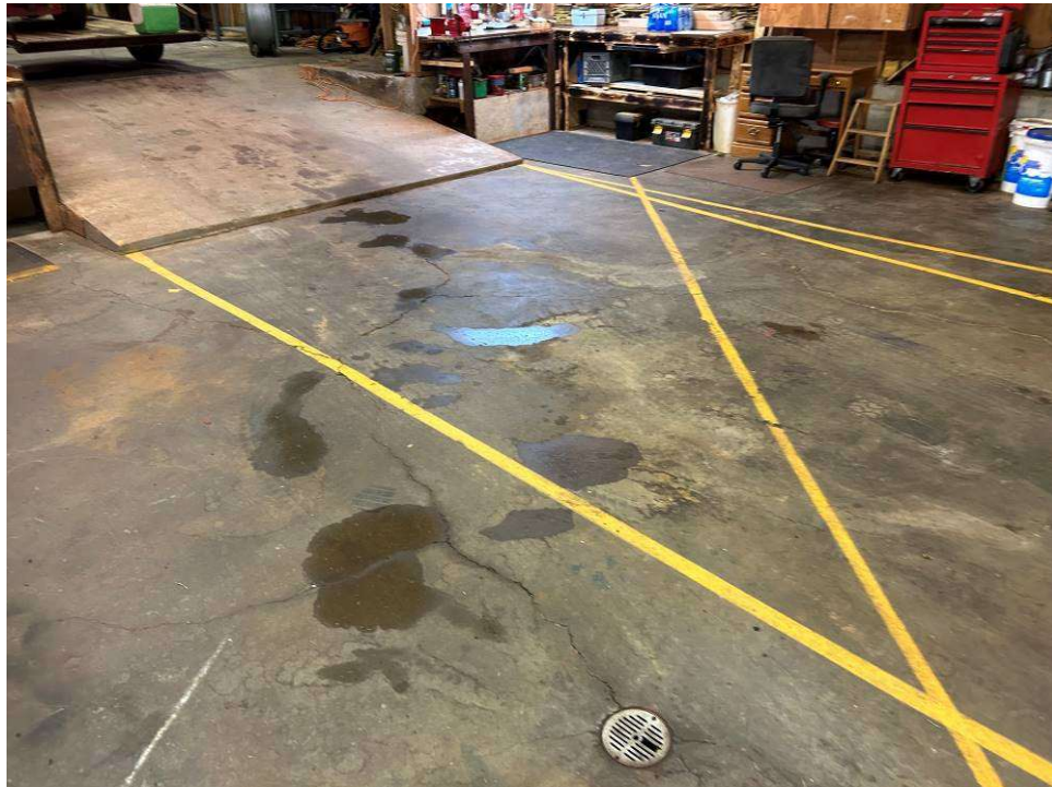
22. View of cracked section of concrete in maintenance building floor.
