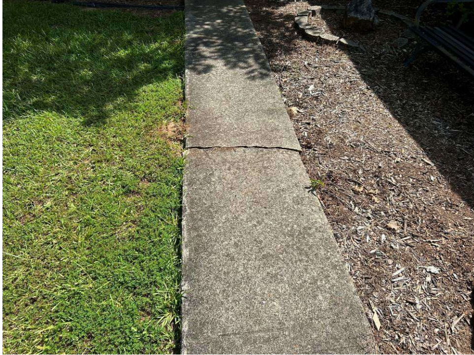
7. View of cracked and settled section of sidewalk.
