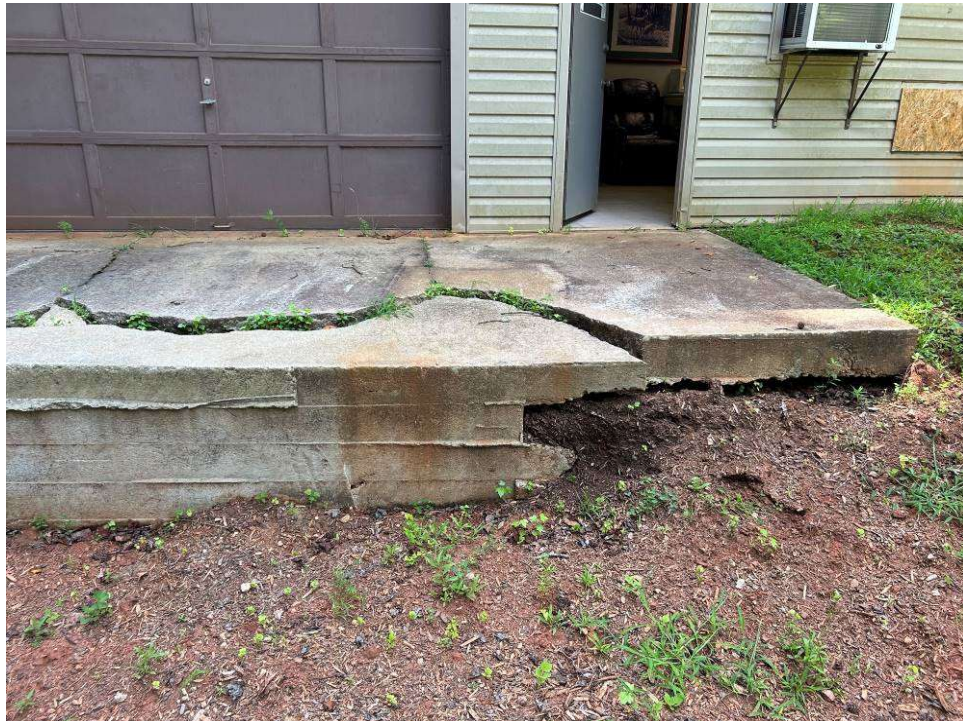
26. View of spalled section of concrete loading dock.
