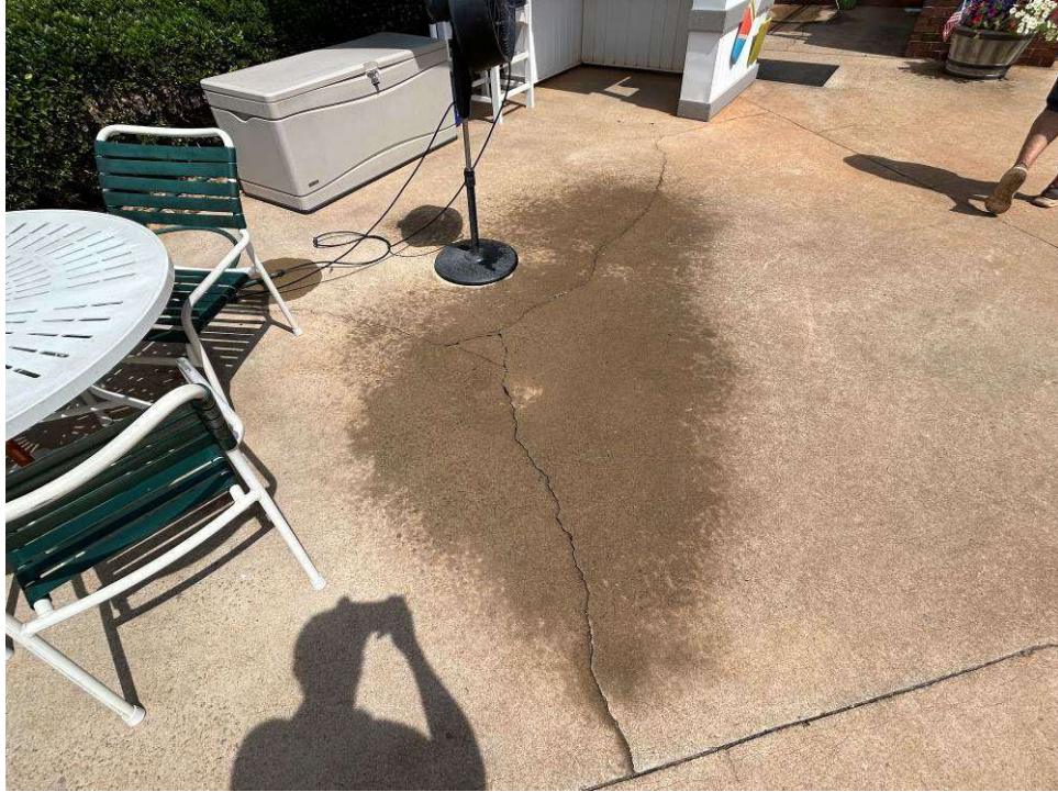
11. View of cracked section of the pool deck.
