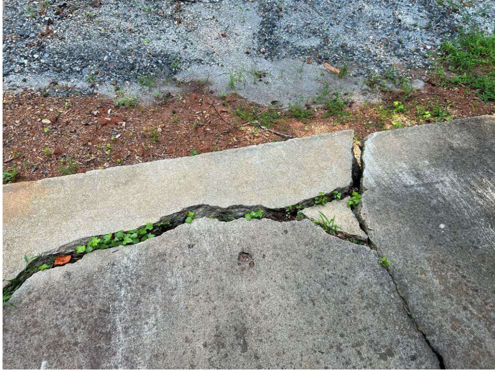
25. View of spalled section of concrete loading dock.
