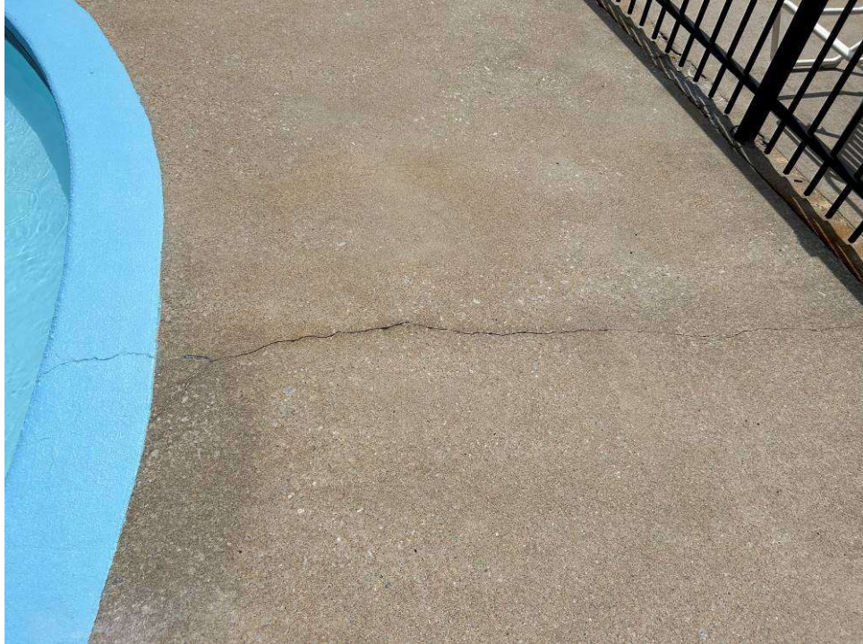
9. View of cracked section of the pool deck.
