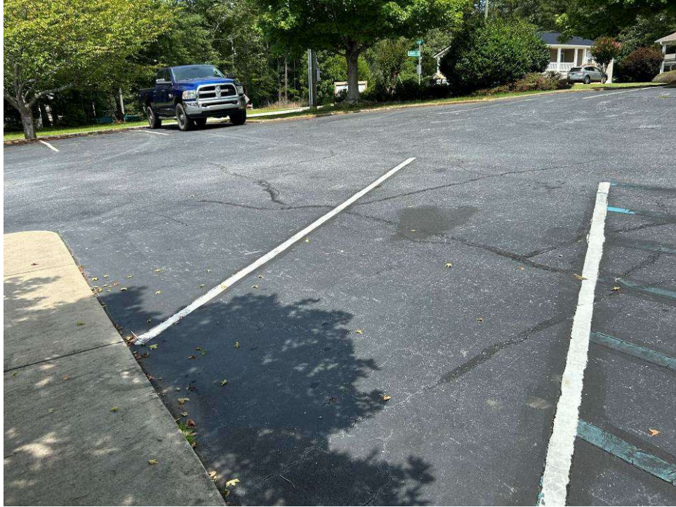
1. View of linear cracks at clubhouse parking lot.
