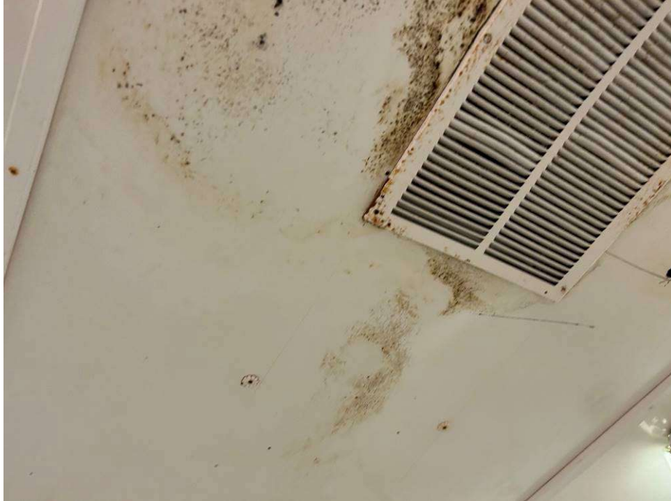
31. View of stains on comfort station bathroom ceiling.
