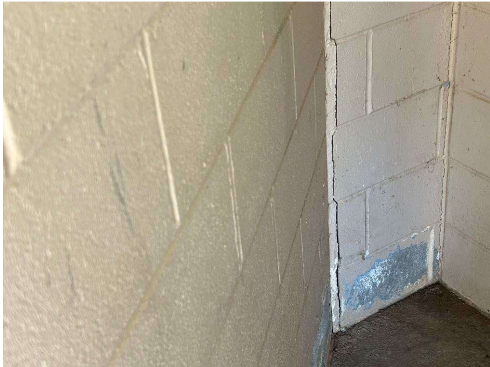
30. View of linear crack in mortar of brick wall at comfort station.
