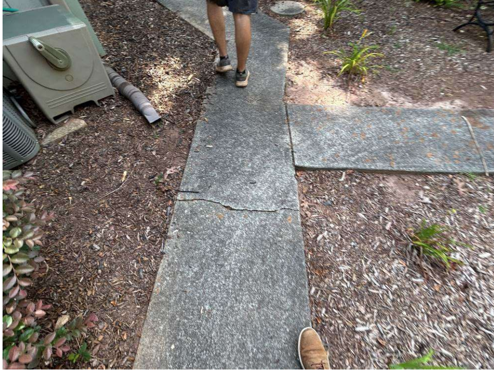
5. View of cracked and settled section of sidewalk.
