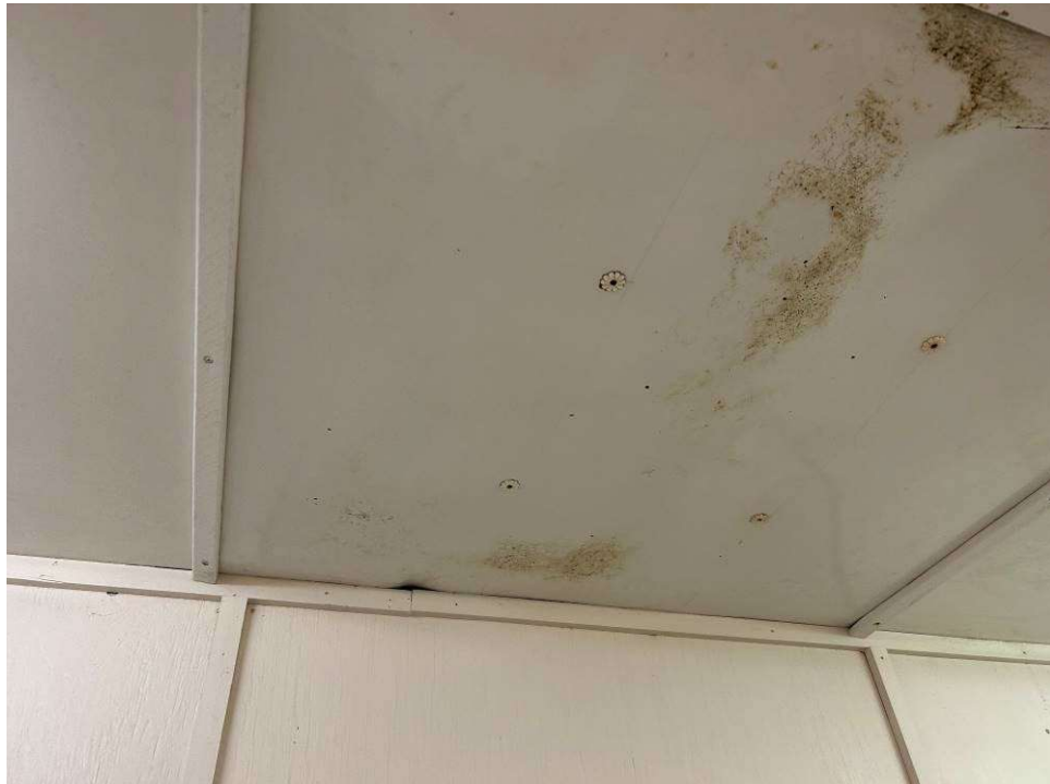
32. View of stains on comfort station bathroom ceiling.
