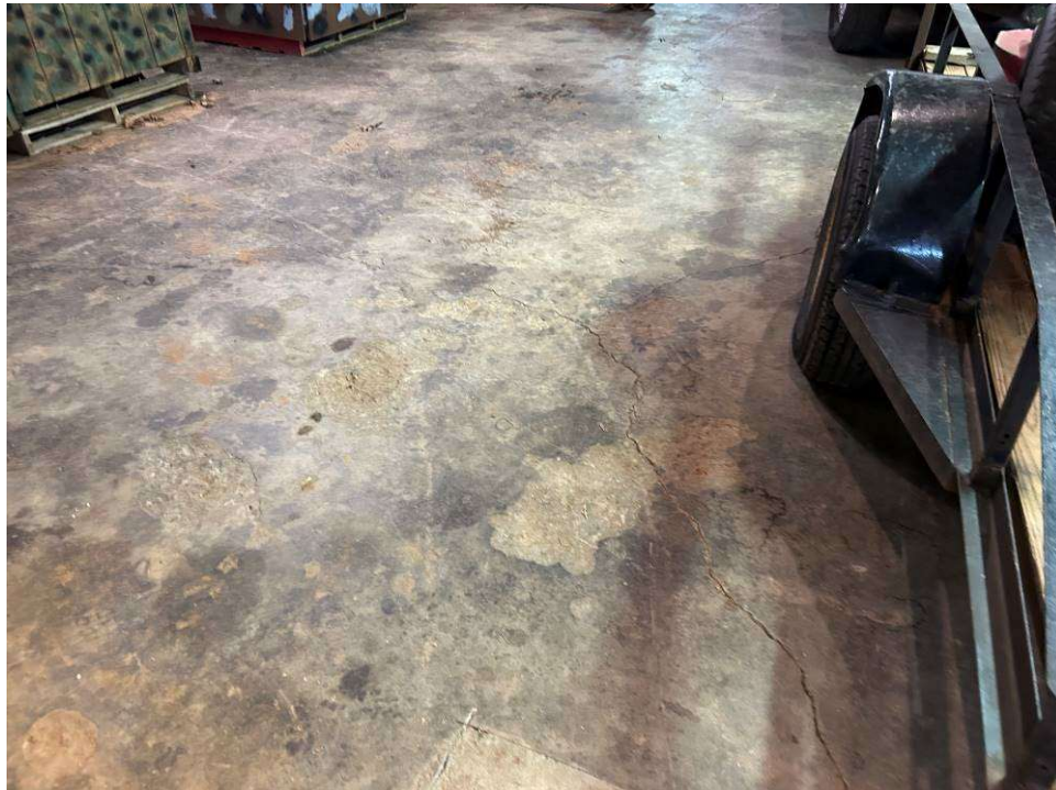
24. View of cracked section of concrete in maintenance building floor.
