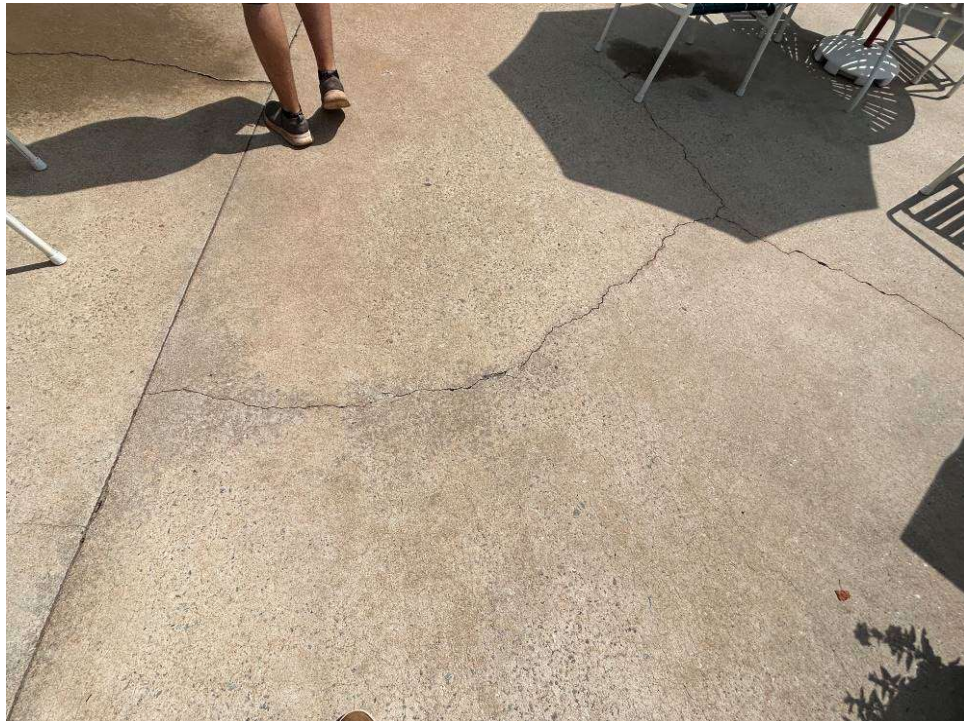
10. View of cracked section of the pool deck.
