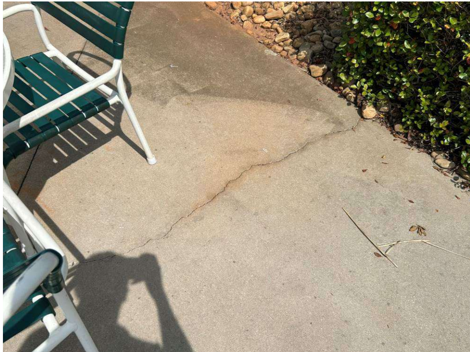
8. View of cracked section of the pool deck.
