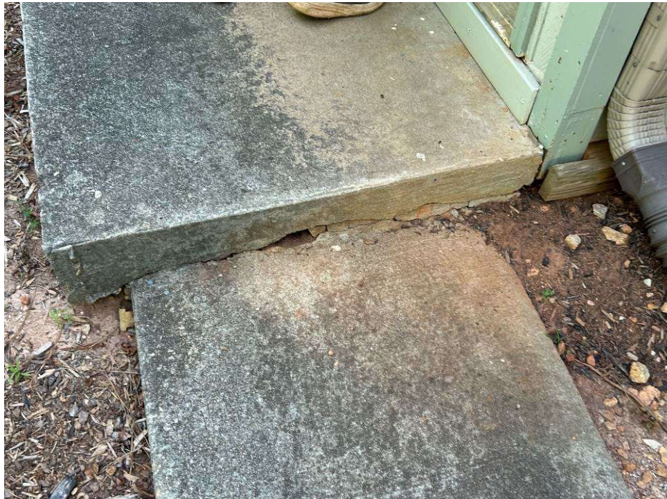
6. View of cracked and settled section of sidewalk.
