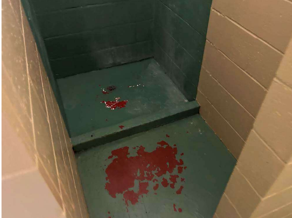
29. View of paint chipping in comfort station bathroom.
