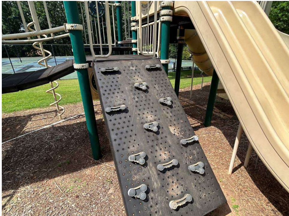
14. View of playground equipment in need of maintenance.
