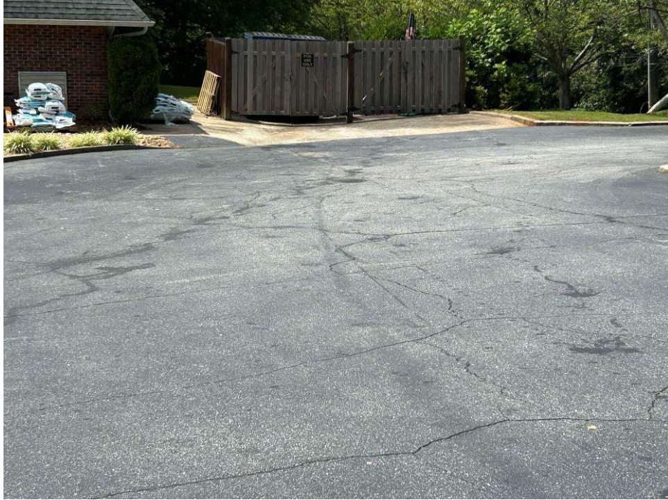
3. View of linear cracks at clubhouse parking lot.
