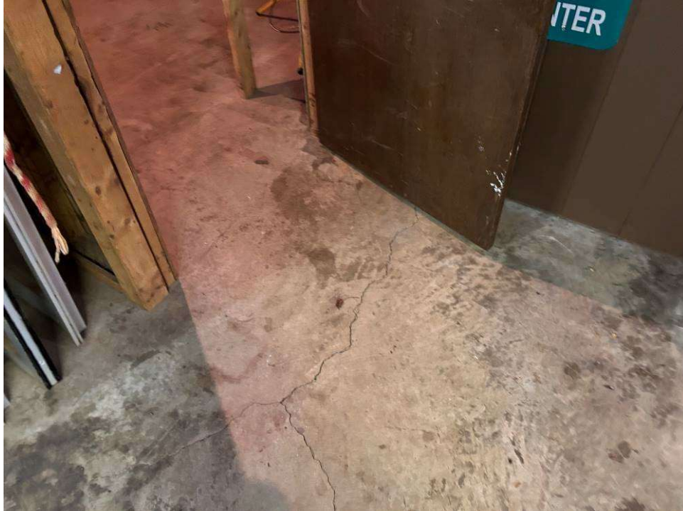
23. View of cracked section of concrete in maintenance building floor.
