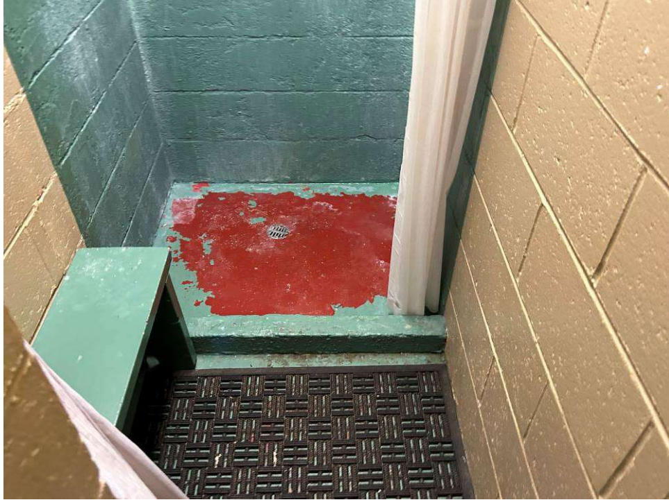
27. View of paint chipping in comfort station bathroom.
